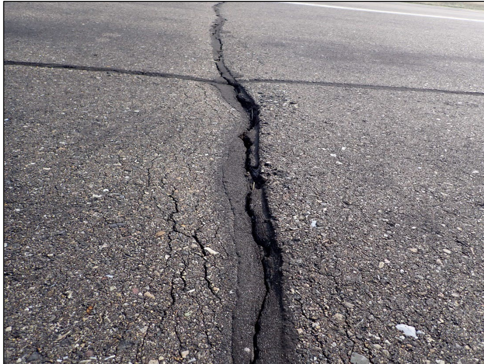
RW02-03-18: L&T Cracking
