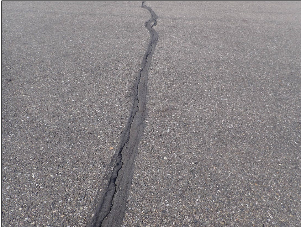
AP-01-21: L&T Cracking
